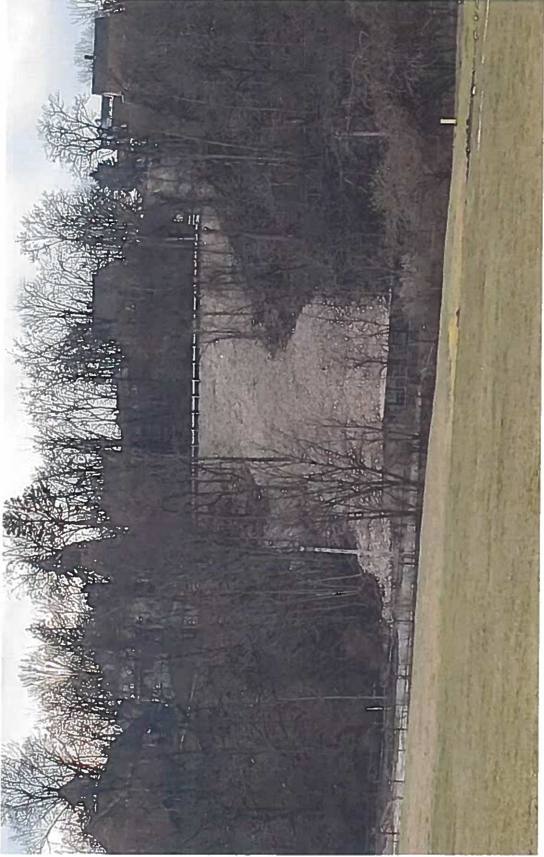
Griffith Slide Repair from Jefferson Ave. Park
